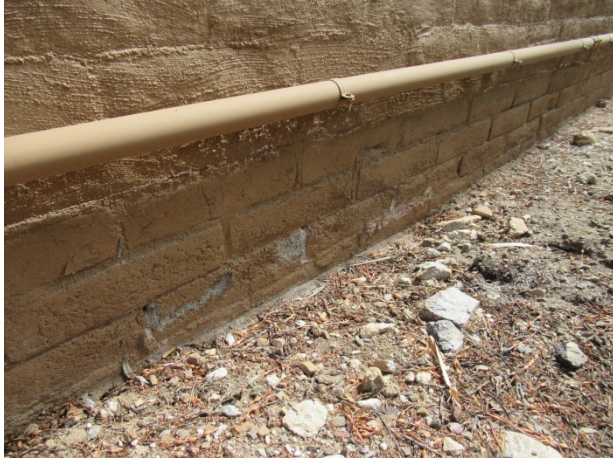
Spalled masonry at base of wall
