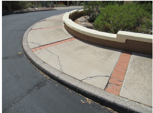
Typical cracks at cul-de-sac island
