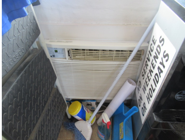
Current HVAC unit at gate house
