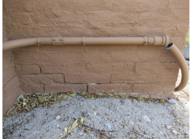
Mortar deterioration at base of wall
