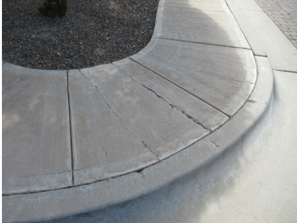
Concrete sidewalk cracks near entrance
