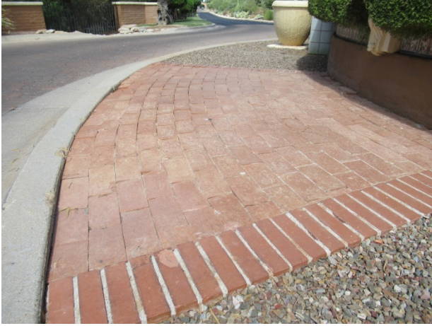
Settlement at pavers adjacent to fountain water feature
