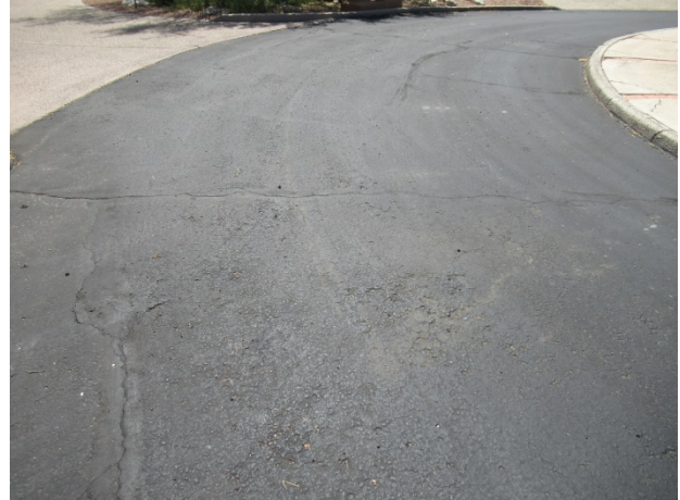
Raveling and cracks at East Cathedral Rock Circle
