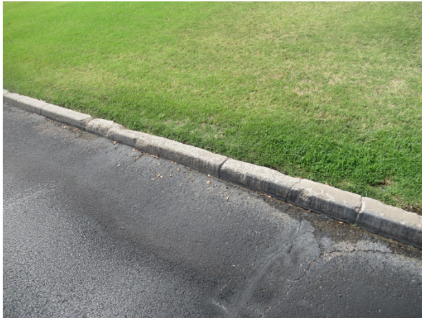
Concrete spalls and cracks near entrance
