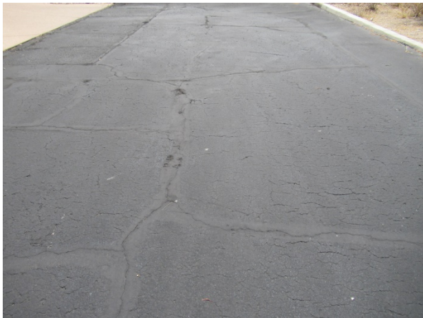
Various cracks at East Finger Rock Road
