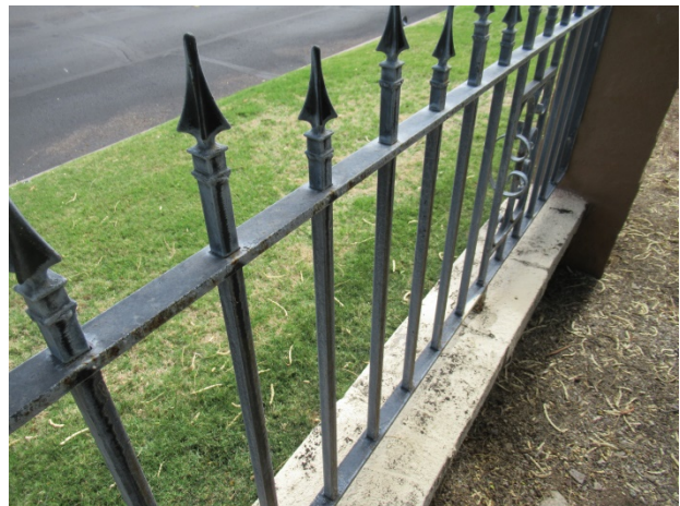
Typical rust and paint deterioration
