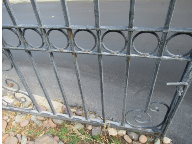
Rust and finish deterioration at decorative gate
