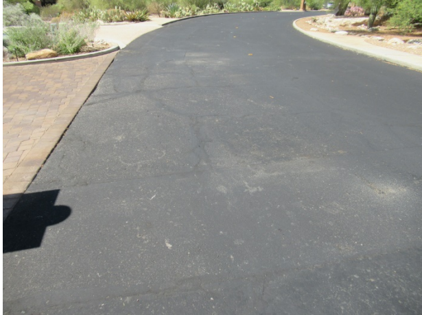
Cracks and edge settlement at North Cathedral Rock Road
