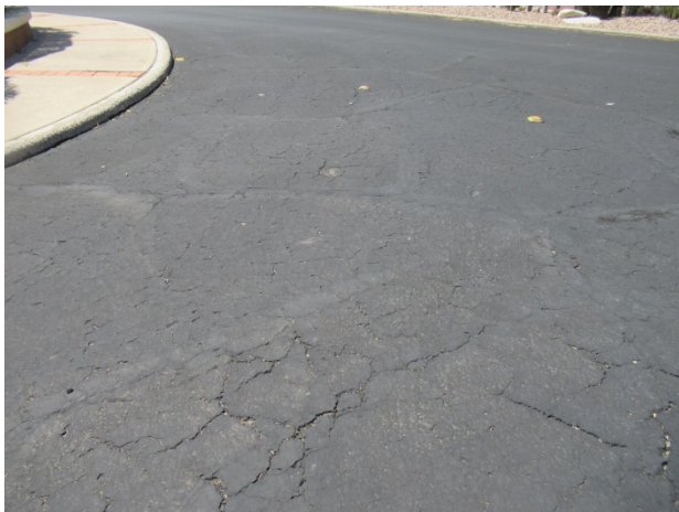
Cracks throughout at East Sun Cloud Place
