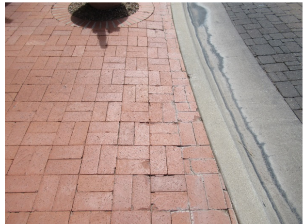
Cracks and spalls
