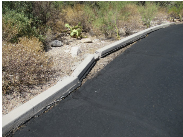
Damaged curb at Window Peak Road
