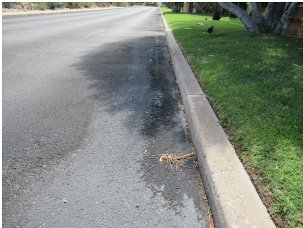
Pavement raveling and standing water at East Ina Road
