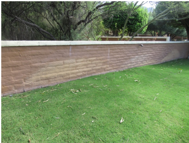
Finish deterioration and efflorescence at perimeter wall
