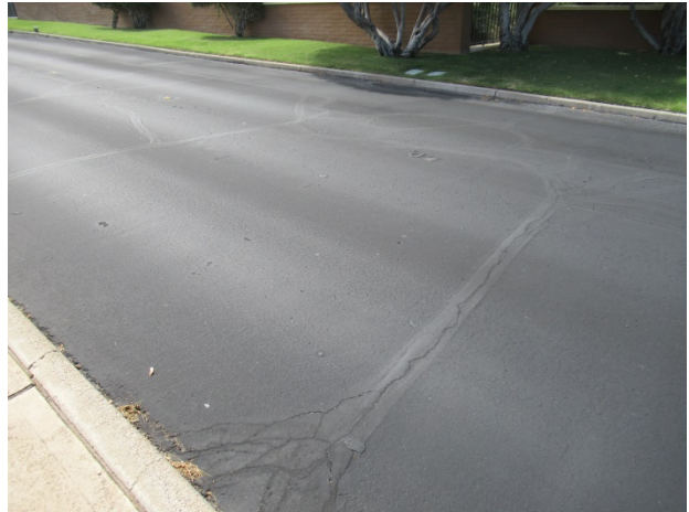
Various cracks at East Ina Road
