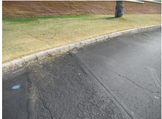
Spalls and cracks near entrance
