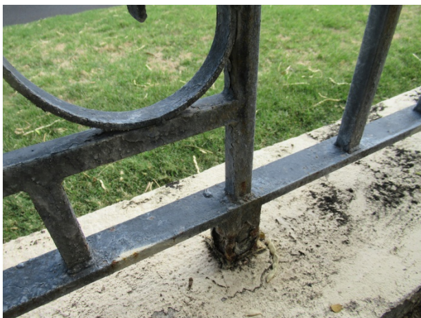
Significant paint deterioration and corrosion at post pocket
