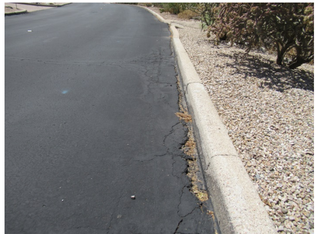
Edge cracks and raveling at North Moon Spirit Lane
