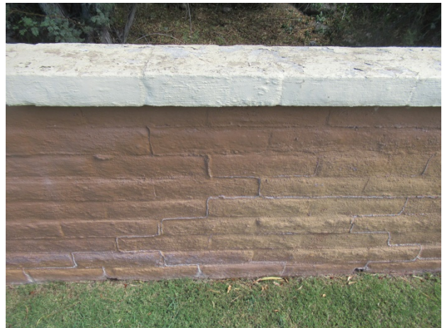
Efflorescence and peeling paint finish at coping
