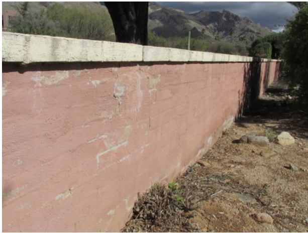
Perimeter wall rear with finish deterioration and cracks
