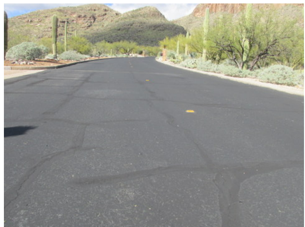
Cobblestone Road overview with block cracks, fatigue cracks, seal coat deterioration and repairs
