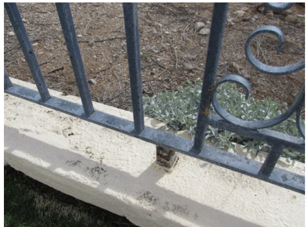
Typical metal fence along perimeter wall with rust and paint finish deterioration
