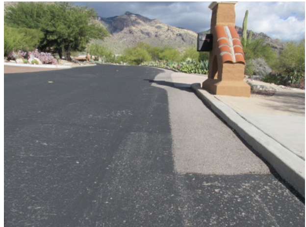
Cathedral Rock Road overview with partial replacements, seal coat deterioration and cracks
