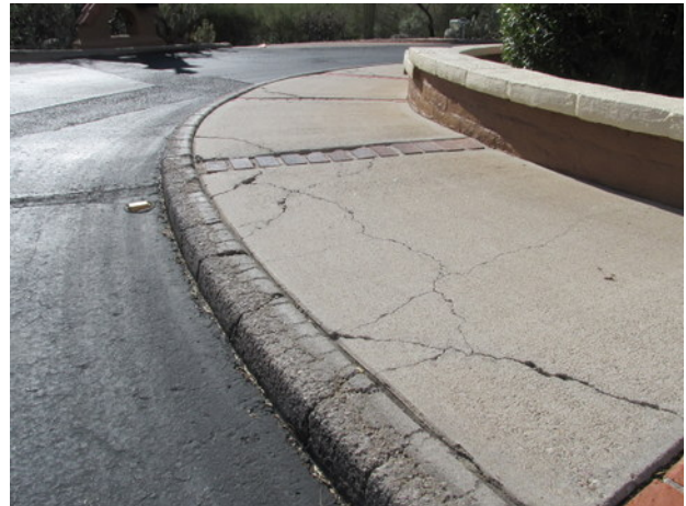
Significant concrete curb and sidewalk cracks and deterioration along Finger Rock Circle
