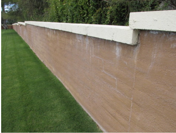
Perimeter wall overview with minor cracks, finish deterioration and efflorescence
