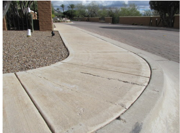
Concrete sidewalk cracks near office building and gate house area
