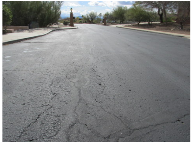
Cathedral Rock Road overview with cracks and previous repairs
