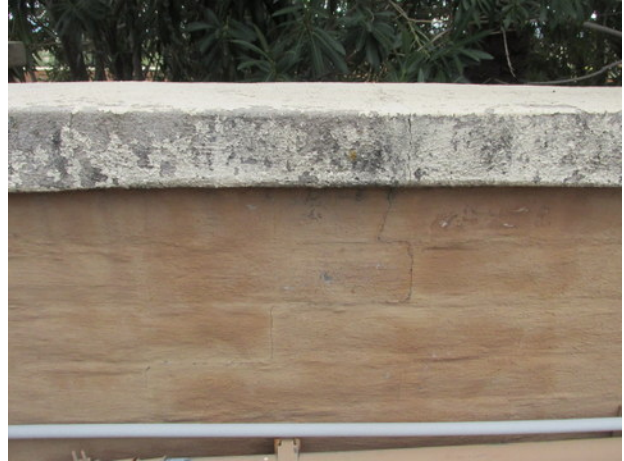
Perimeter wall coping cracks and finish deterioration
