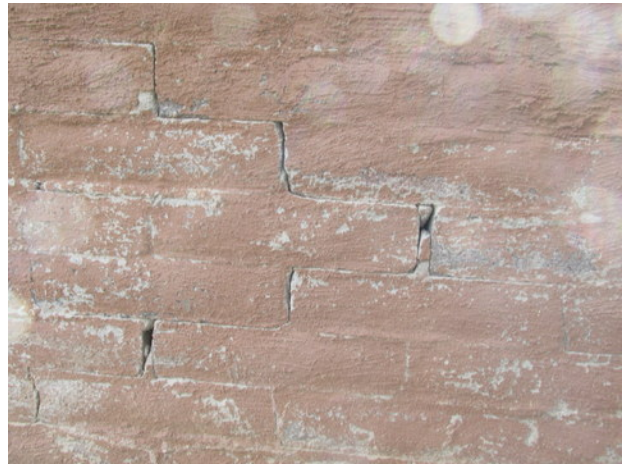
Perimeter wall finish deterioration, cracks and mortar deterioration
