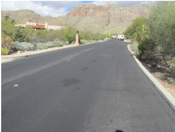
Cobblestone Road overview with vehicle fluid stains, seal coat deterioration, cracks and previous repairs
