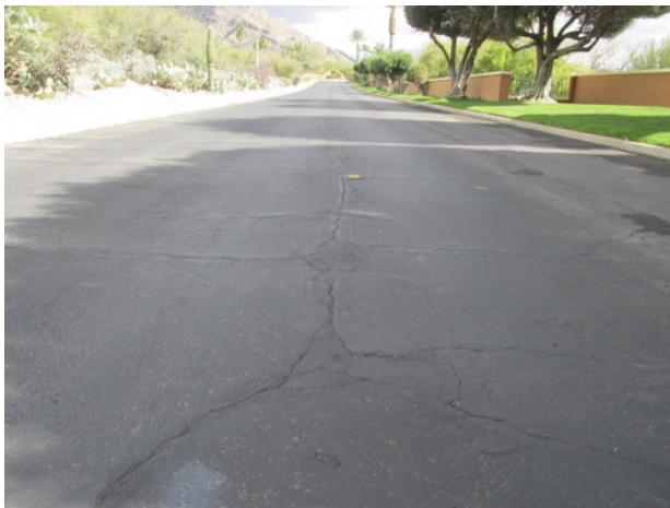
Ina Road overview with block cracks, previous repairs and seal coat deterioration
