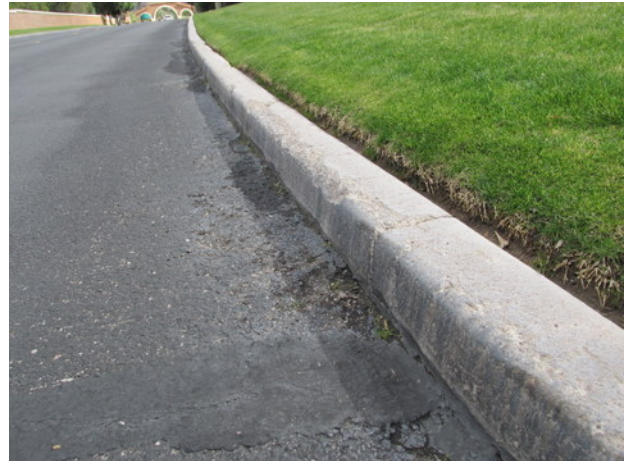
Concrete curb spall along Ina Road
