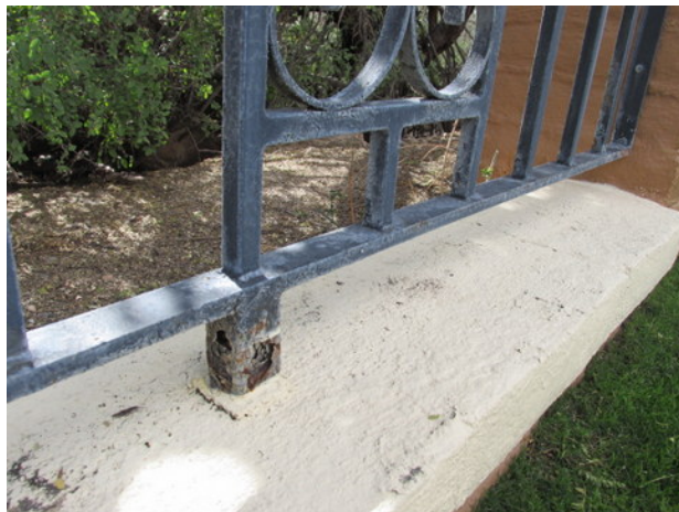
Typical metal fence along perimeter wall with rust and paint finish deterioration
