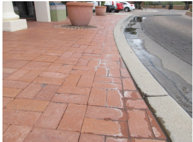
Masonry pedestrian pavers at office building with settlement, efflorescence and standing water
