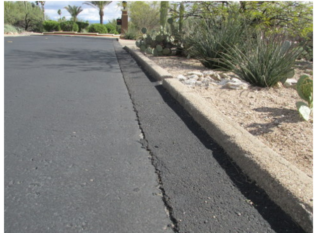
Windsong Place overview with cracks, seal coat deterioration and partial replacements
