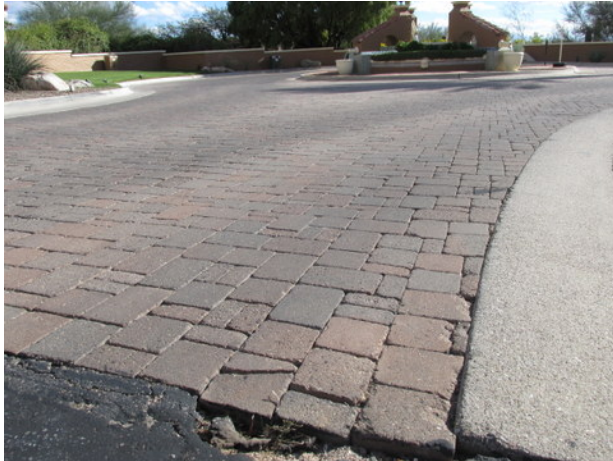
Masonry pavers near Cobblestone Road with minor cracks and settlement
