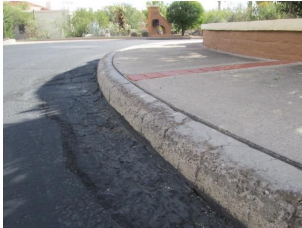
Significant concrete curb cracks and spall along Sun Cloud Place
