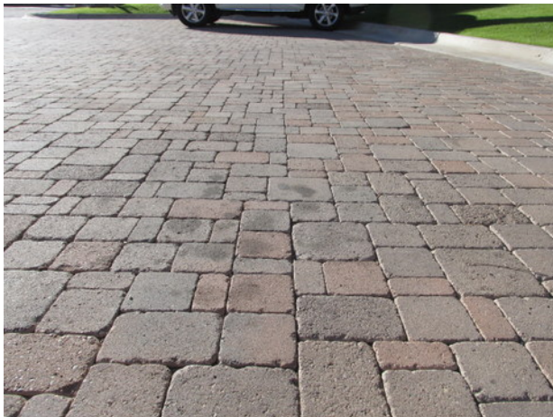
Masonry pavers near office building with vehicle fluid stains
