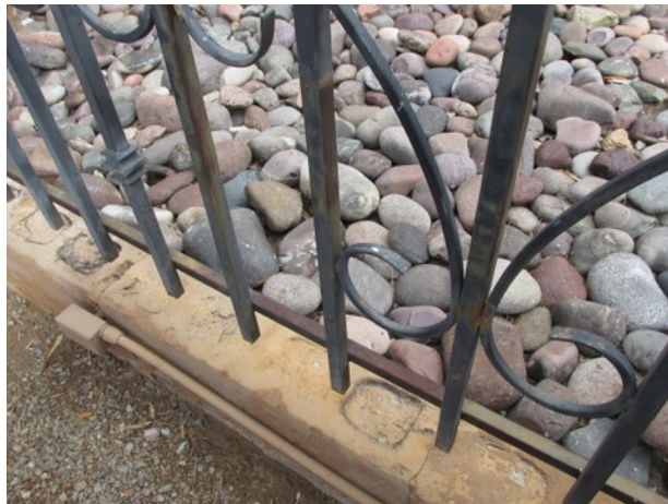
Decorative community entrance gate with rust and paint finish deterioration
