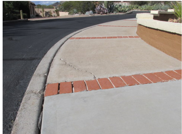
Concrete sidewalk cracks along Star Fury Place
