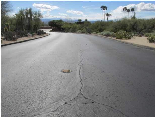
Catalina Ridge Drive overview with cracks and previous repairs
