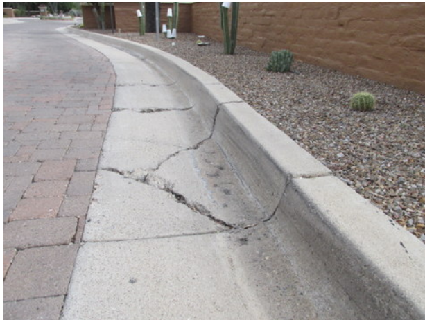
Concrete curb and gutter cracks and deterioration near gate house
