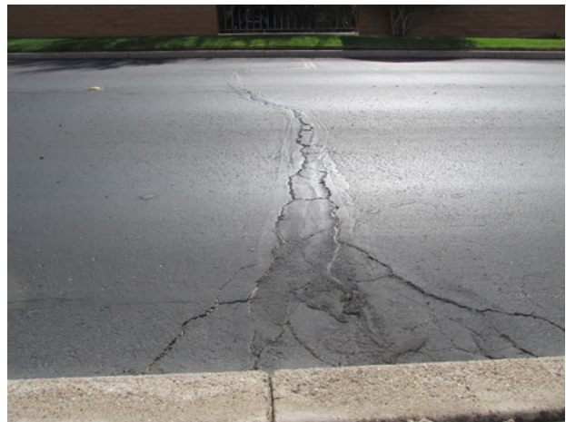
Ina Road with lateral cracks and previous repairs
