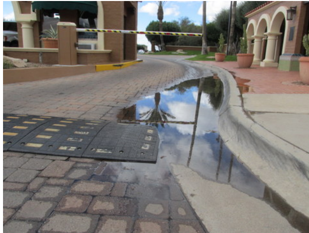
Standing water at pavers and concrete gutters near office building
