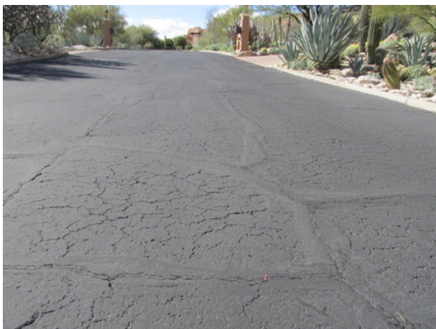
Finger Rock Road overview with block cracks, fatigue cracks and previous repairs
