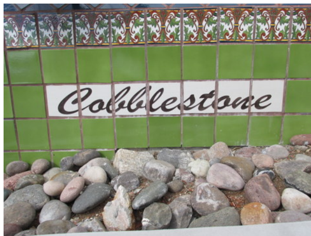
Typical monument tile with minor finish deterioration
