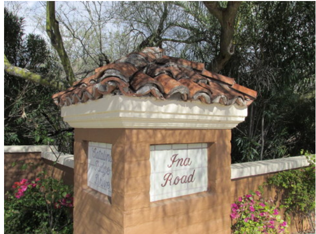
Monument at street entrance with concrete tile roof deterioration
