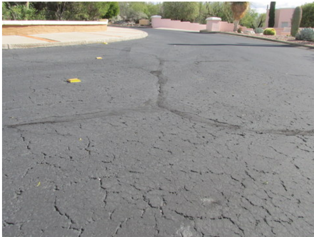
Sun Cloud Place overview with previous repairs, seal coat deterioration and fatigue cracks
