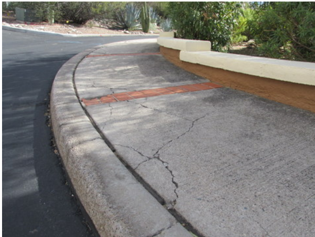
Concrete sidewalk cracks and deterioration along Moon Spirit Place
