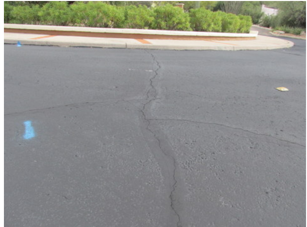
Moon Spirit Place overview with transverse cracks and previous repairs
