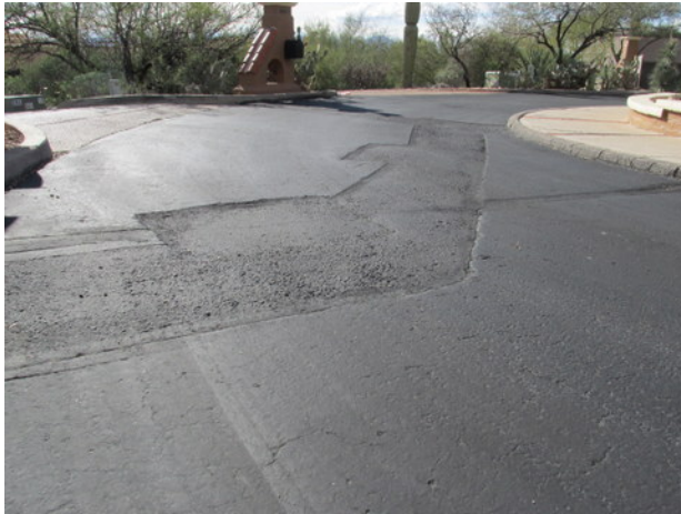
Finger Rock Circle overview with partial replacements, previous repairs and cracks
